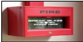
Emergency Break Glass
